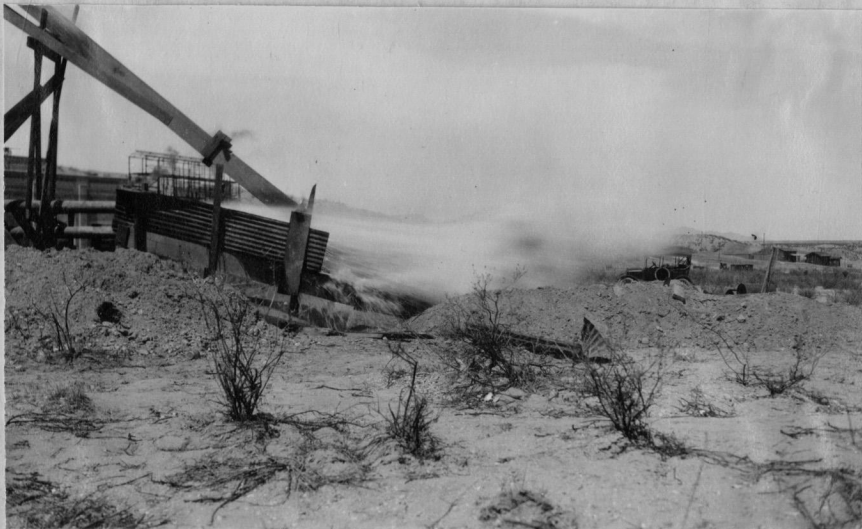
Fig. 24.- Developing and testing a well with air lift. The air valve was opened quickly throwing a spray of water out 75 to 100 feet horizontally.
