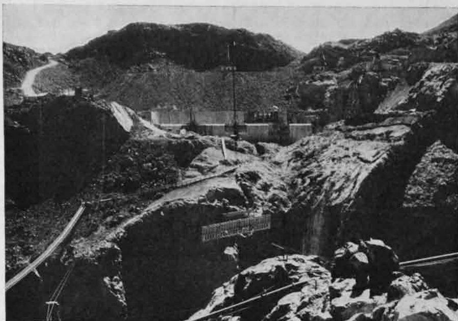
A network of cableways swings high over the gorge. This one and its mate, both of the traveling type, serve the two spillways and the upstream portion of the dam.
