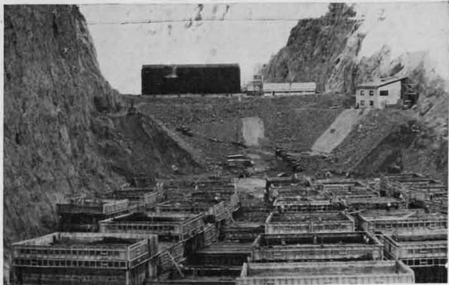
Refrigeration equipment for cooling of 3,400,000 yd. of concrete in Boulder Dam is located at bottom of the canyon just below the dam. Cooling tower for first stage of heat dissipation is shown at top center, located on the downstream cofferdam. After storage has commenced in the reservoir, this cooling tower will be dismantled. Refrigeration plant can be seen against canyon wall at extreme right.
