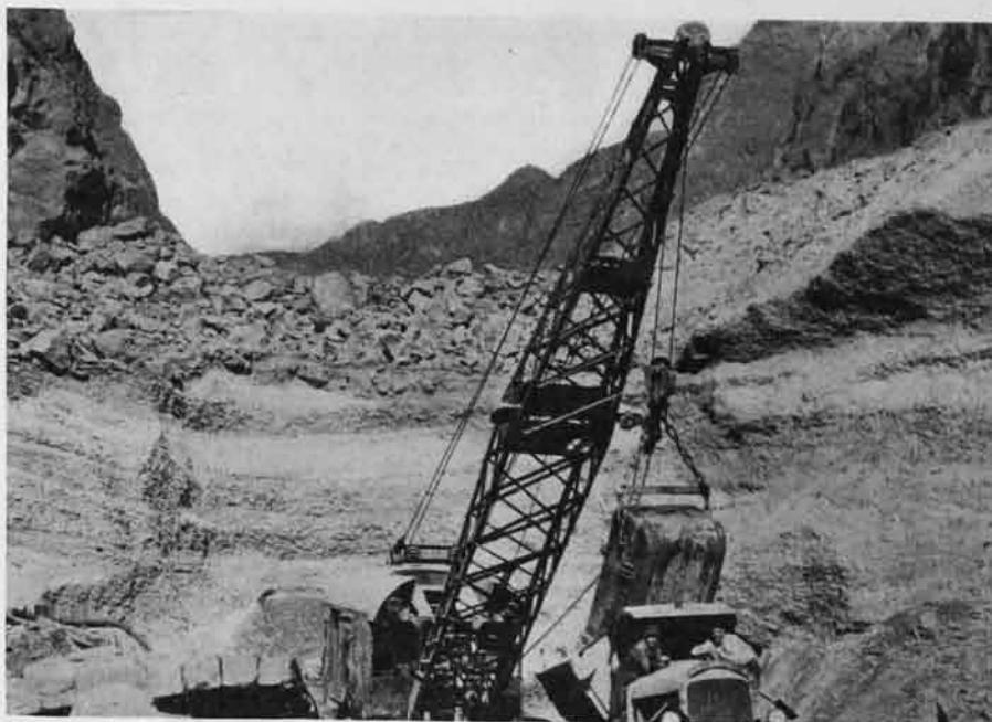
Fig. 1—River fill at dam site proved to be compact, tight and remarkably stable, providing ideal foundation for cofferdams. Stratification of sand and gravel layers is well illustrated by this view. Broken rock on top of fill is from canyon-wall scaling.
