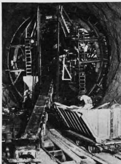
Fig. 4—Belt conveyor carries concrete into steel-form section in lining sides and invert of the 37-ft. upper penstock headers. Arch lining is placed with pneumatic guns.
