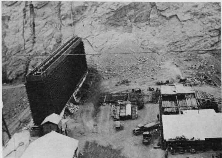
The cooling tower and header pipe yard, located on the crest of the downstream cofferdam, as seen from the Nevada wall of the canyon.
