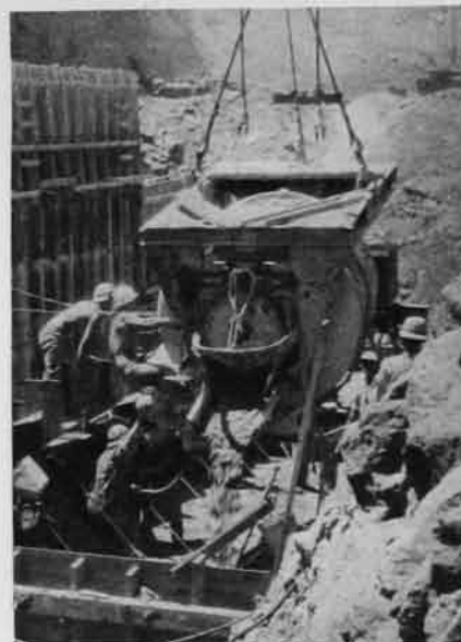
Fig. 7—In the confined space of the abutment blocks that are not up to the full size, the buckets are too difficult to handle and concrete is placed with 4-yd. agitators.
