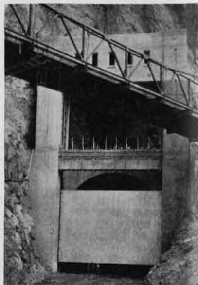
Fig. 5—Stoney gate on the downstream portal of the inside diversion tunnel on the Nevada side.
