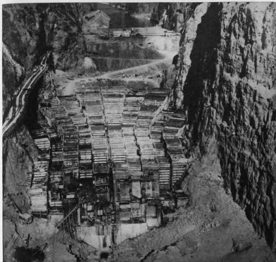
Fig. 1—Foundations of the barrier that will block the Colorado. About 32,000 cu.yd. of concrete are required for each 5-ft. lift of the dam at this stage of construction. Concrete reaches the dam via the double-track railroad hugging the left canyon wall. Five cableways distribute concrete to the forms in 8-yd. buckets.
