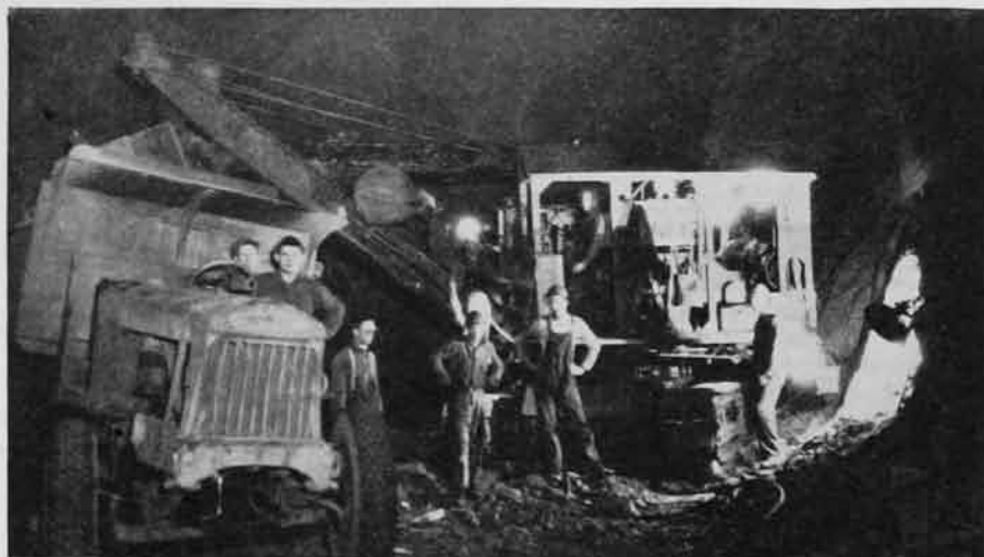
Fig. 2—Muck in 37-ft. penstock tunnels is handled with electric shovels and trucks. These tunnels start at vertical curve from the bottom of intake towers and end in a group of small outlet tunnels. They were driven from adits.
