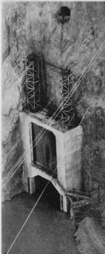
Fig. 6—Steel bulkhead gate in position at the upstream portal of the outside diversion tunnel on the Arizona side. This gate and a similar one on the other side will be lowered only once into final position to start storage in the reservoir. Low flow in the river permits a temporary cofferdam to make the other tunnel available for trucking.
